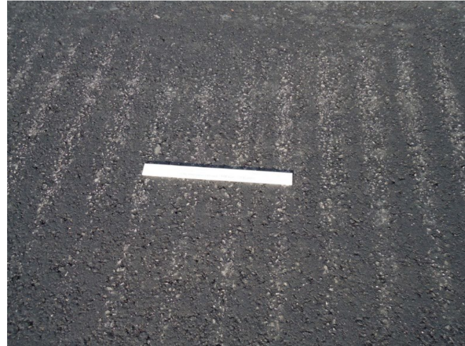
Over or Under- Compaction Can Occur
