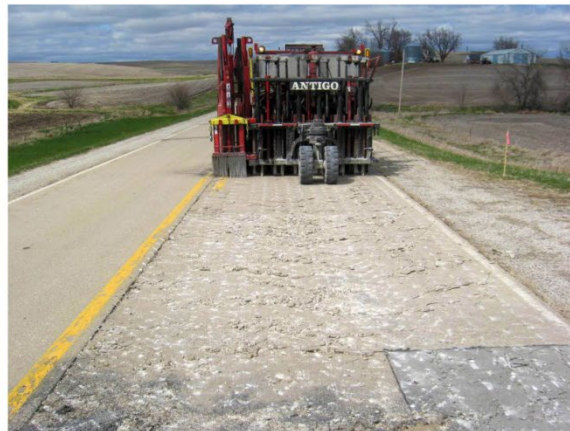
Modified Rubblization—significant spalling
